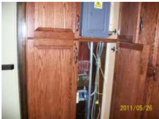
The electrical cabinet which provides access to the switches as well as to the circuit breakers.
