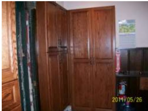
The cabinets at the southwest corner of the sacristy. The cabinet on the left houses the electrical panels and the cabinet that is facing front is for clergy and server vestments.
